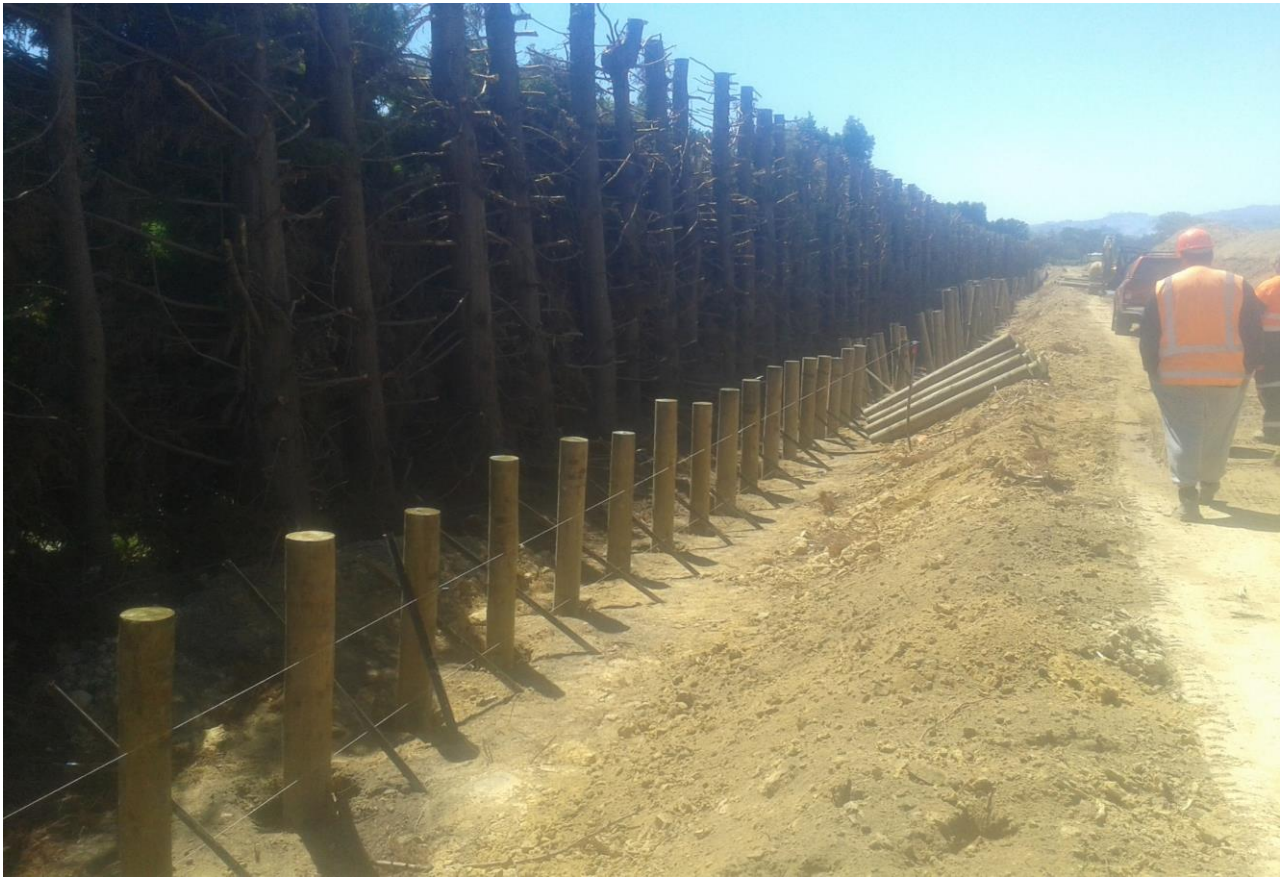
Photograph 3: Photo taken on the 22/11/16 of the final placement and alignment of retaining wall piles.
